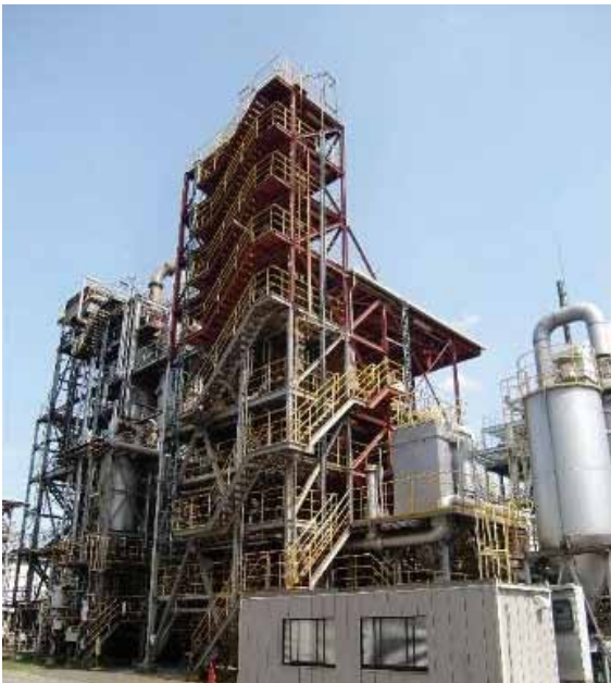
Figure 4 Over view of CFB boiler pilot facility
