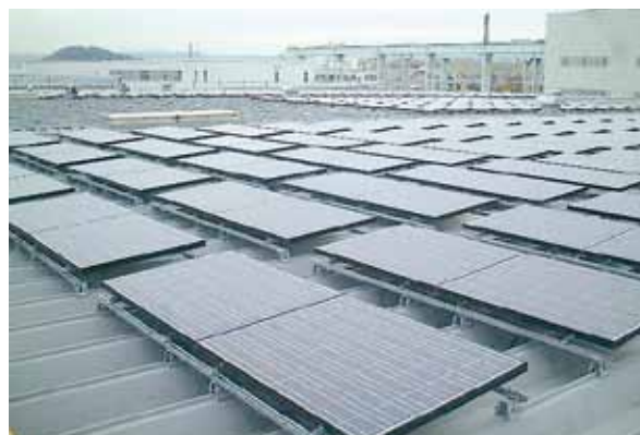
図6 横須賀製造所精密機械棟 太陽光発電設置状況 Photovoltaic power generation at precision machinery building in Yokosuka factory
